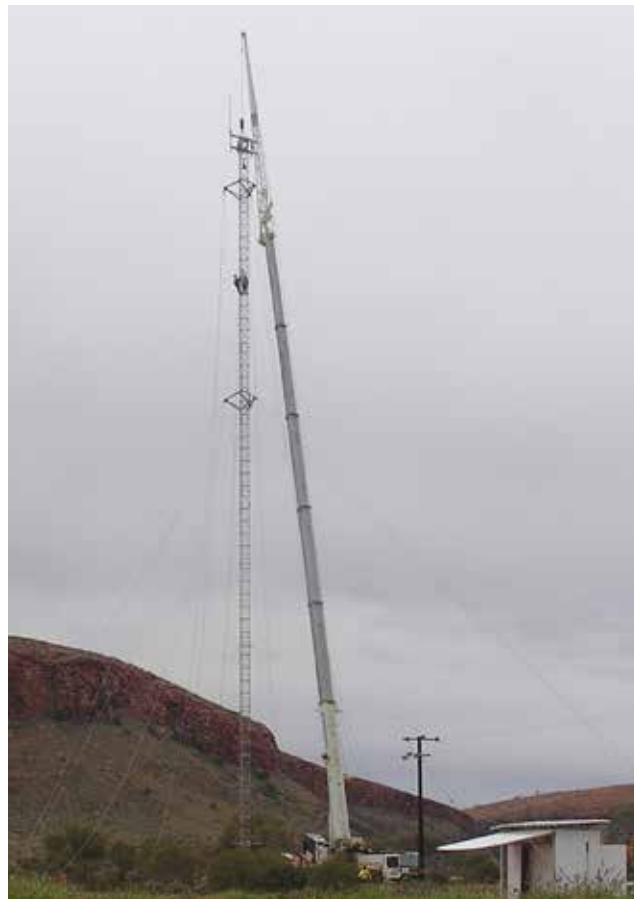
New mobile tower being installed a Warakurna Community on the Ngaanyatjarra lands
