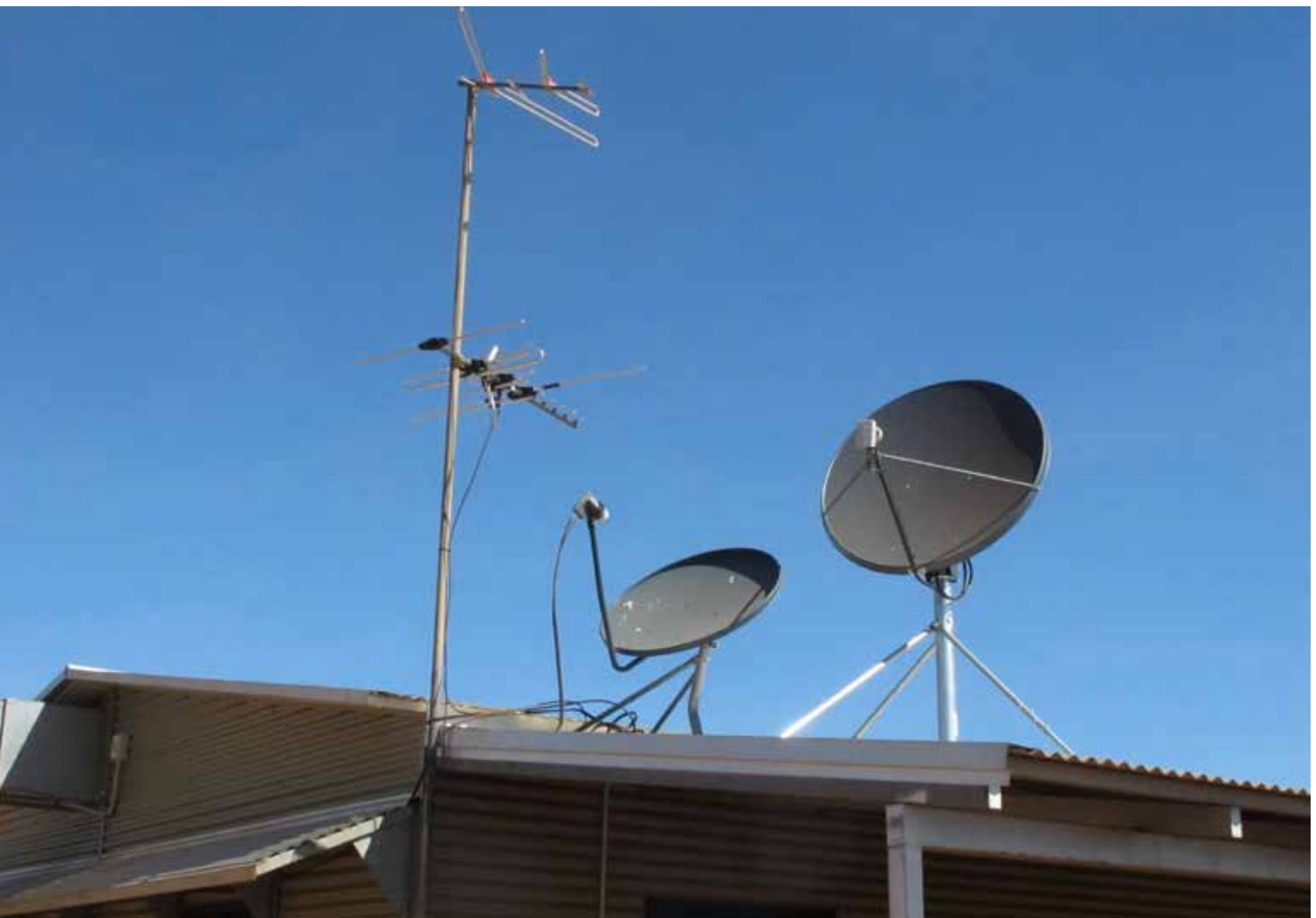
Below: Switchover infrastructure being rolled out across remote Australia
